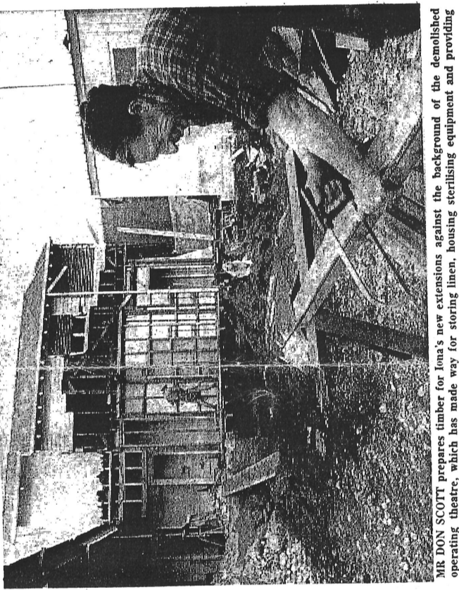
MR DON SCOTT prepares timber for Iona's new extensions, against the background of the demolished operating theatre, which has made way for storing linen, housing sterilising equipment and providing a sewing room.
