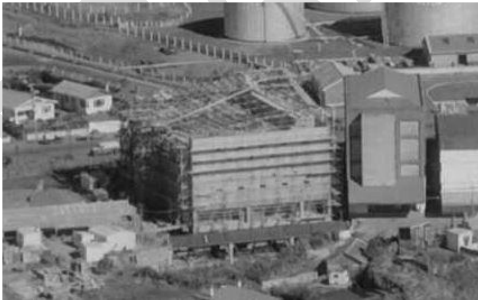
Parsons Store under construction, 22 August 1958. Detail from Whites Aviation aerial photograph, Whites Aviation Collection, Alexander Turnbull Library, WA-47172-F.
