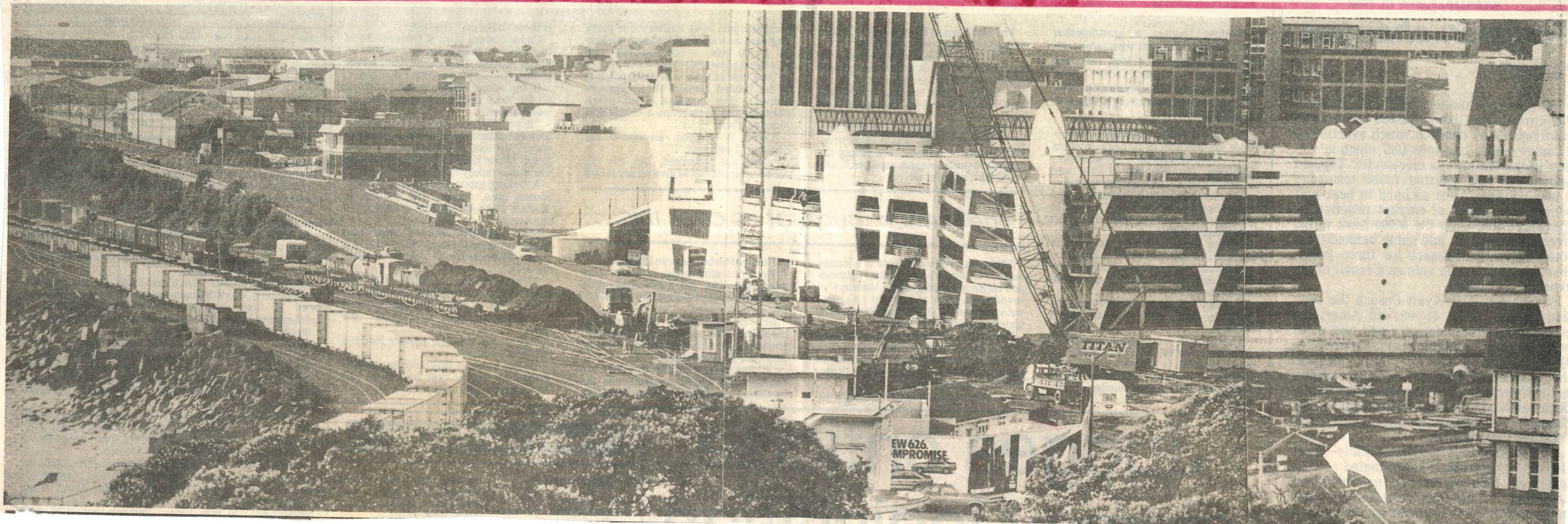
New Plymouth's newest section of roadway slowly wends its way west, past the Centre City shopping centre. The roadway will eventually pass over a new bridge before joining St Aubyn St at the area indicated by the arrow.
