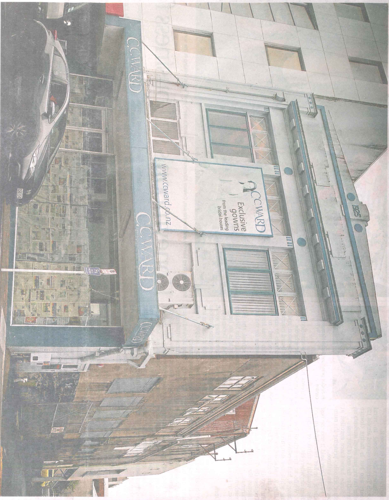
The old C.C. Ward building in Currie St, New Plymouth, is sealed off, having been declared 'dangerous' by the district council.
