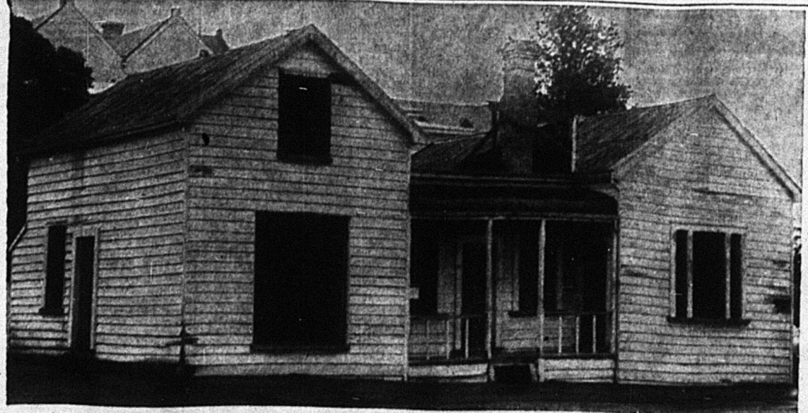
MAKING WAY for New Plymouth's new courthouse building, one of the city's oldest wooden houses is now being demolished. Familiarly known as the "grog" shop, it has associations with the regiments engaged during the Maori Wars. It fronts on to Silver Street, which is to be closed at some future date.
