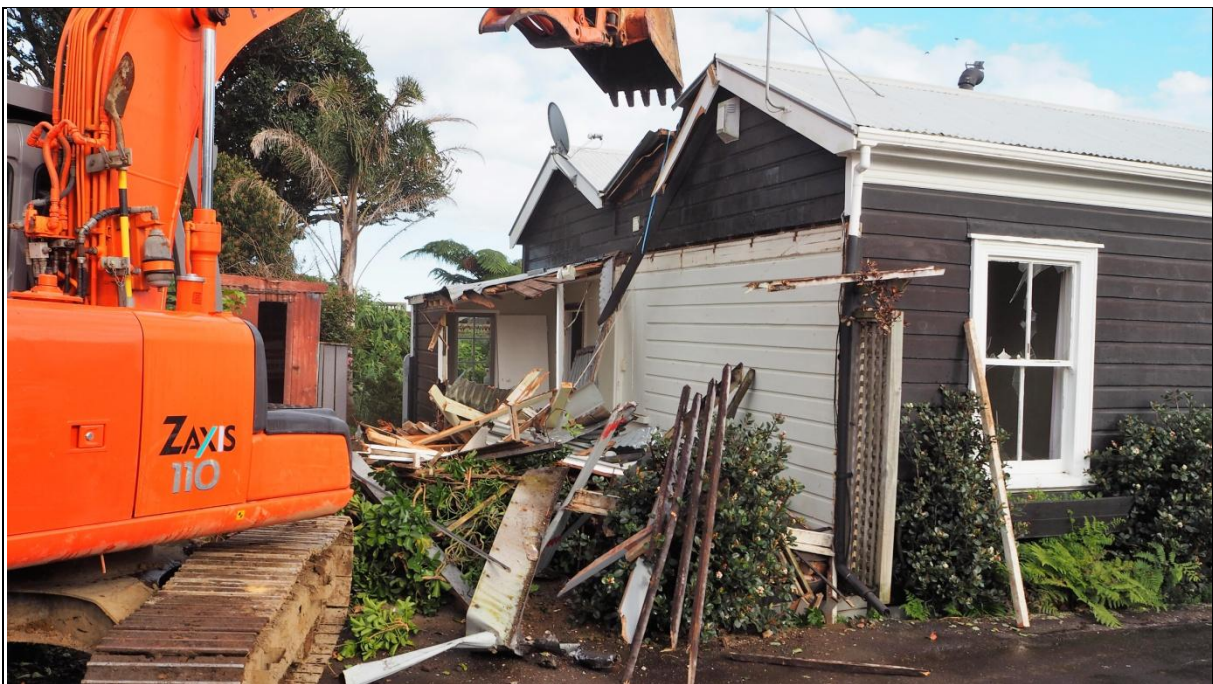
Figure 10: The rear addition partially demolished, showing the original weatherboard cladding below the western gable that was later enclosed by the lean to addition. Some form of rear addition was always a part of the building, as the roof rafters for the roof of the structure are notched into the studs of the rear wall, creating a gap between the
