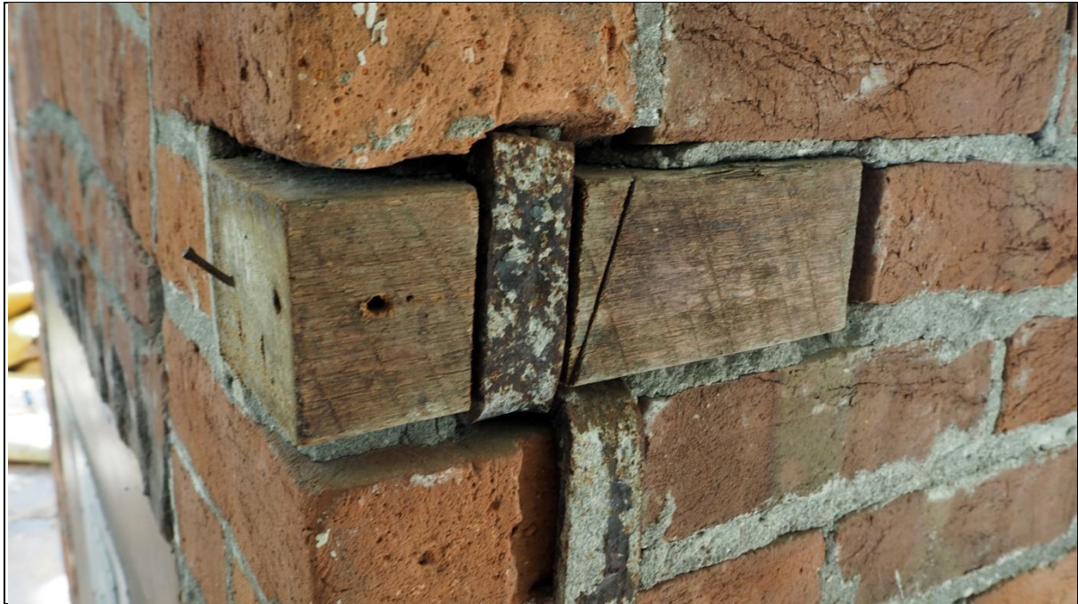
Figure 36: In-situ iron lintel exposed in the corner of the fireplace. The timber surround may have allowed for mantelpiece attachment. Image: Ivan Bruce, 2017.
