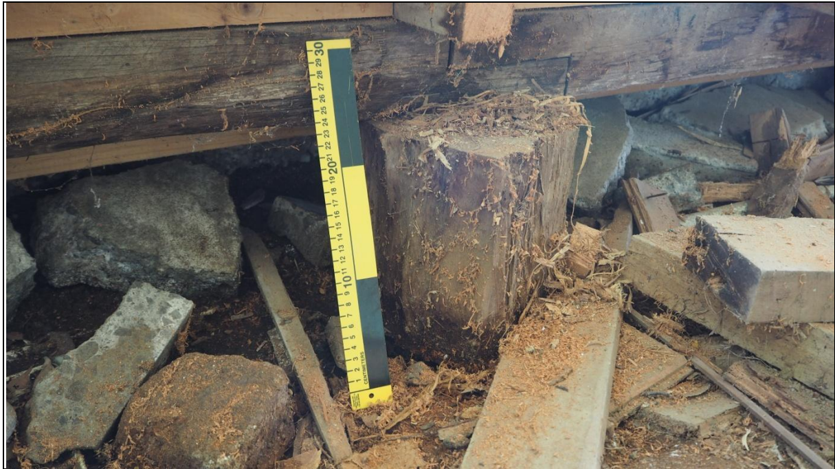
Figure 19: Totara pile below the eastern wall of the cottage. Note the bearer is lapped and joined at the pile. Image: Ivan Bruce, 2017.
