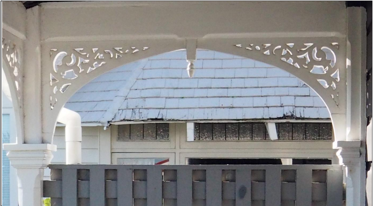
Figure 16: Western end of the veranda, showing the detail of the veranda posts and capitals, pendants and brackets with decorative fretwork. Image: Ivan Bruce, 2017.
