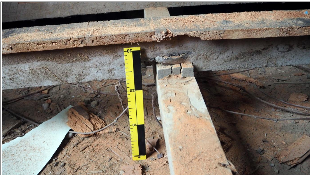
Figure 19: Bearers and joists note this joist has been rebated and then later repacked (possibly following recent re-piling). Image: Ivan Bruce, 2017.
