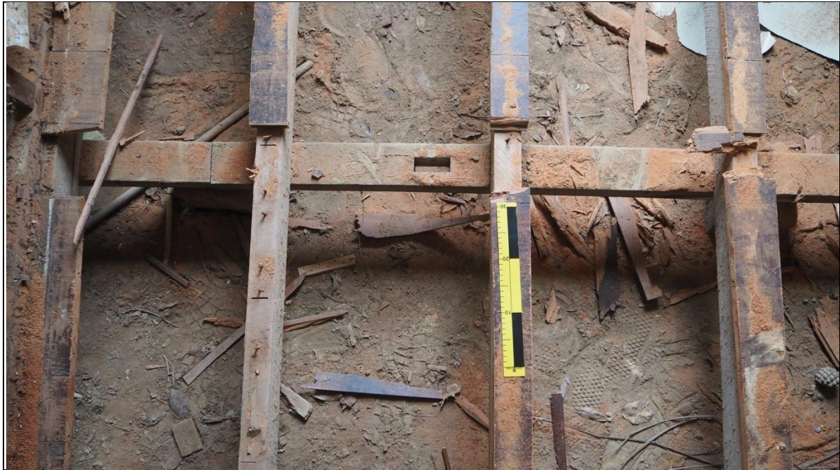
Figure 20: Bearers and joists photographed from above, note mortise in the bearer. Image: Ivan Bruce, 2017.
