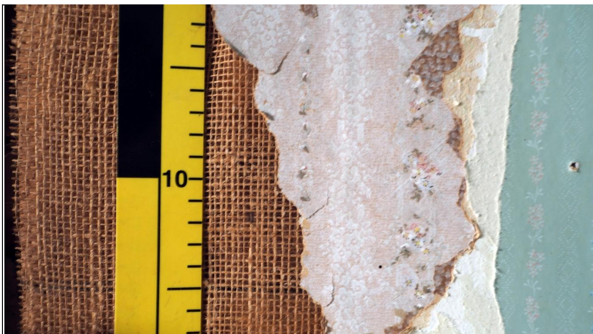
Figure 31: Layers of wall coverings from original sarking cloth covered by wall paper, with sequences of later of wall paper overlaid. Image: Ivan Bruce, 2017.
