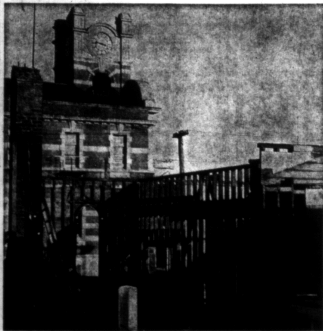
THE AUSTRALIA AND NEW ZEALAND BANK LTD's 91-year-old building on the corner of Devon and Robe Sts, New Plymouth, is slowly disappearing. Today the demolition firm was smashing down the walls. A spokesman for the squad said today it had been difficult to remove about 60 kauri studs. The floor had to be ripped up to get them out. The demolition is expected to be finished by Thursday. The bank is making way for a £67,000 building for MacEwans Machinery Ltd.
