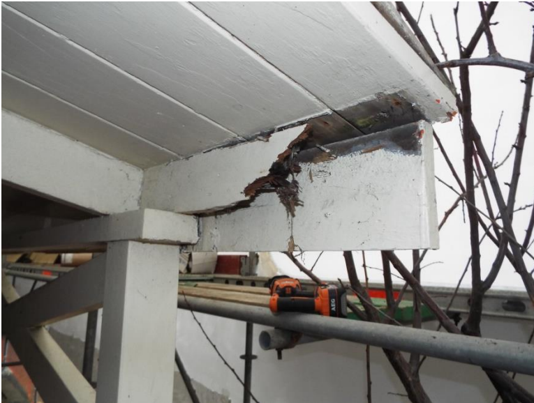
Remedial work required to verandah beam
