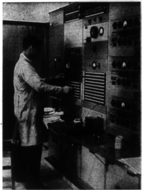
THIS SWITCHBOARD is an essential part of New Plymouth's communication with the outer world for it provides the outlet for the teleprinter and the means of connections to the outgoing parts of Taranaki served from New Plymouth as their main office. A telegraph mechanic adjusts the wires during testing of the new board.
