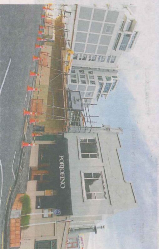
Two industrial buildings from the 1920s have come down on Gill St to make way for a motel.
