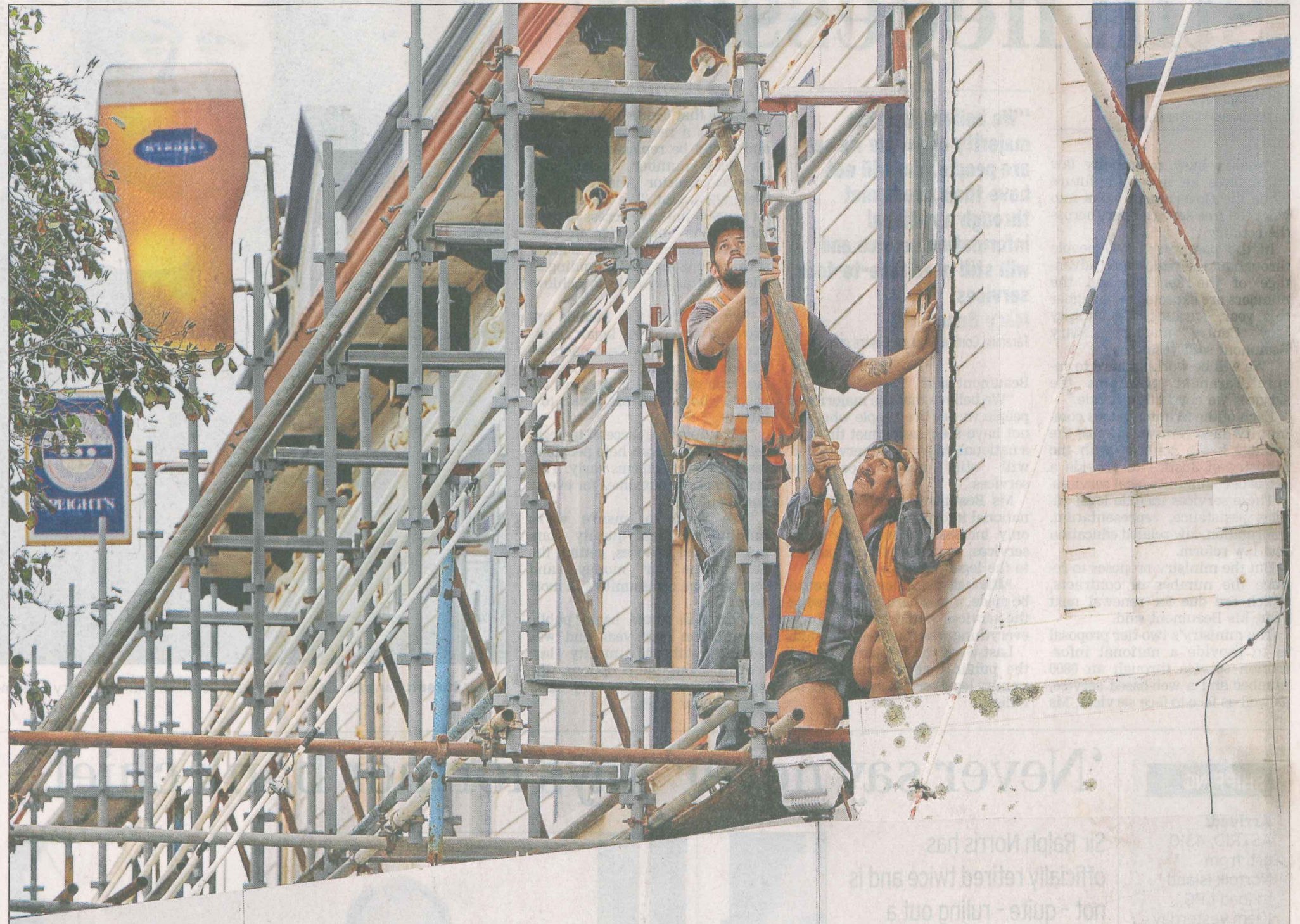
Makeover: The old State Hotel Burton's on the corner of Devon St East and Eliot St is being transformed by the Macfarlanes Group and Garageworks into a Joe's Garage. Over the past week scaffolding has been put up around the building in preparation for a paint job. Photo: ROBERT CHARLES/FAIRFAX NZ
