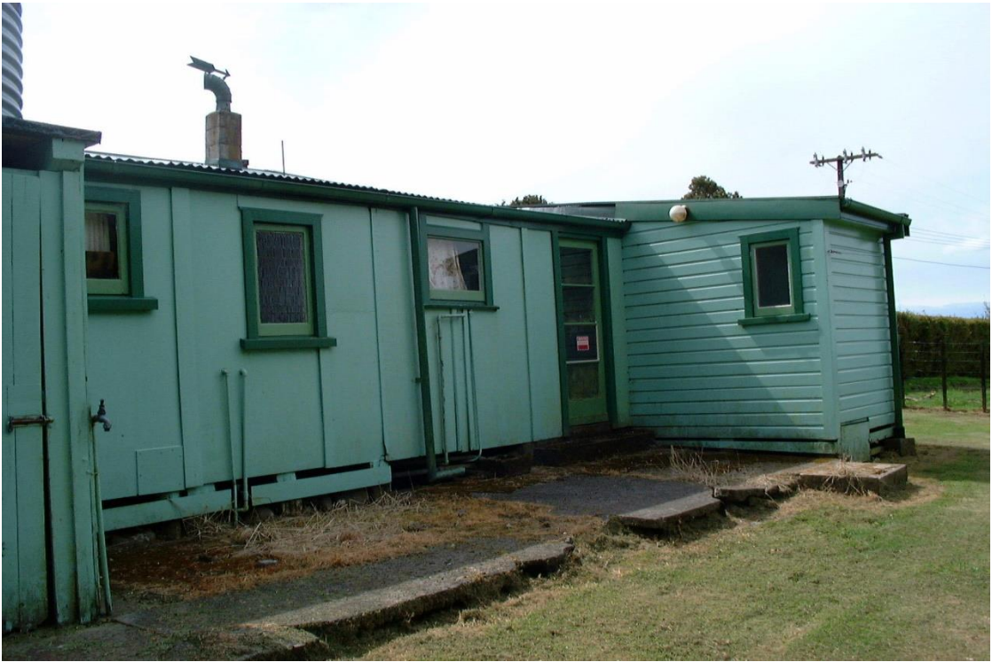
Figure 9: Rear (western elevation) of Rahiri Lodge prior to 2003 upgrade works, Elizabeth Cox, Heritage New Zealand, 4 November 2000.
